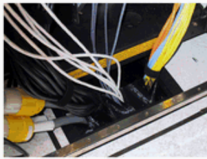
Koldlok tile inserts for airflow management
