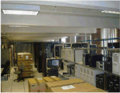
ACI computer room- Before
