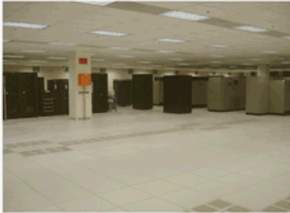
IBM computer room - After
